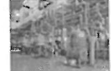
A piping network in an industrial facility. Courtesy of LAMM Engineering, Consulting and Training. Used by permission.
